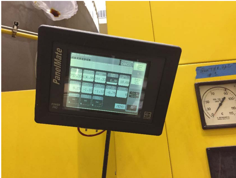
Photo 5. Monitor blade angle digital readout to verify minimal or no blade movement.
